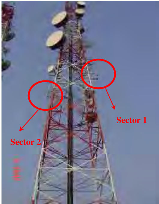
Antennas sector 1 and sector 2
